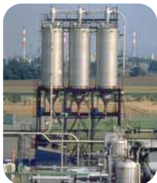
Storage at the Mont plant (Pyrénées-Atlantiques, France)
