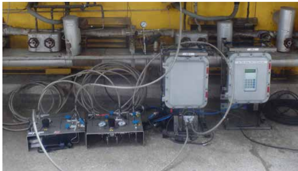
Figure 1 Arkema's H 2 S analyser implemented on site
