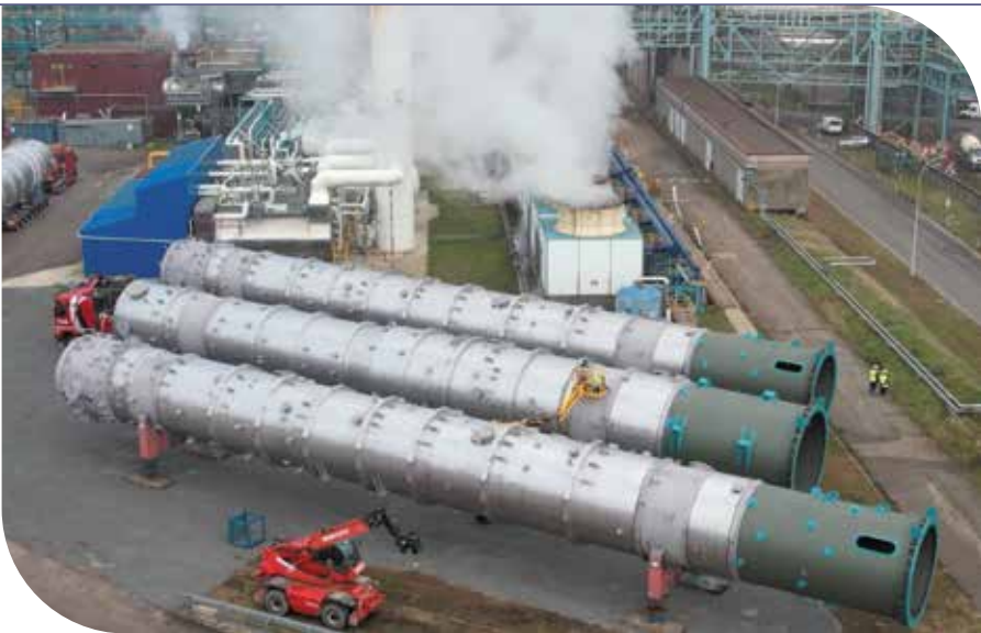
Arkema is investing approximately €130 million in its acrylics facility in Carling, France, to reduce emissions by 20% and ensure the long-term sustainability of its facilities.
